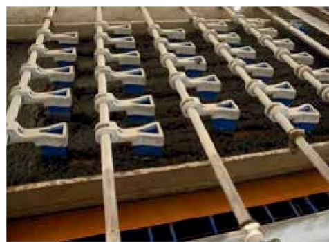
Waste Water Sludge De-Watering
