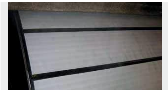
Drum filter with Frame-Trak™
