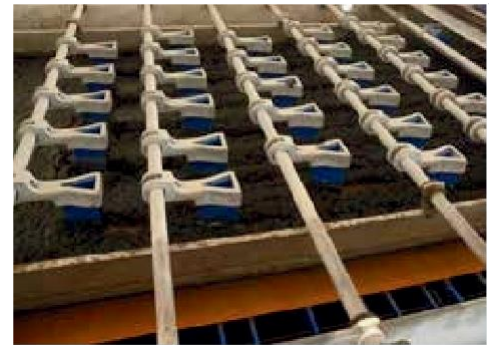
Waste Water Sludge De-Watering
